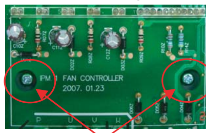
Check assemble condition
