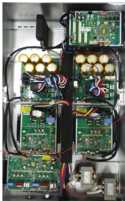
15V Input power wiring conditions
