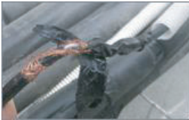
Wiring Fault Case
